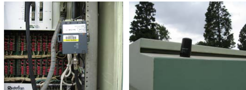
Figure 11-8: Terminal Server and Cabinet-Mounted Antenna
