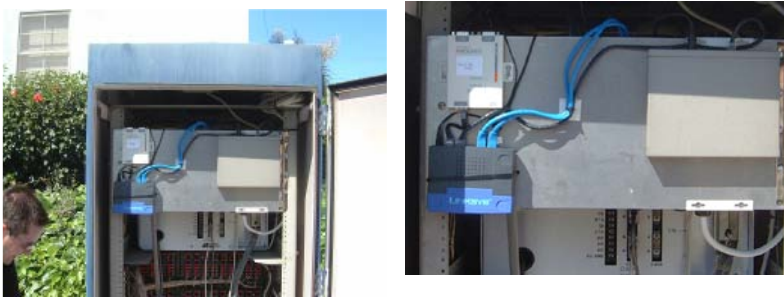
Figure 11-7: AP/Bridge Equipment Panel In Type 332 Traffic Cabinet
