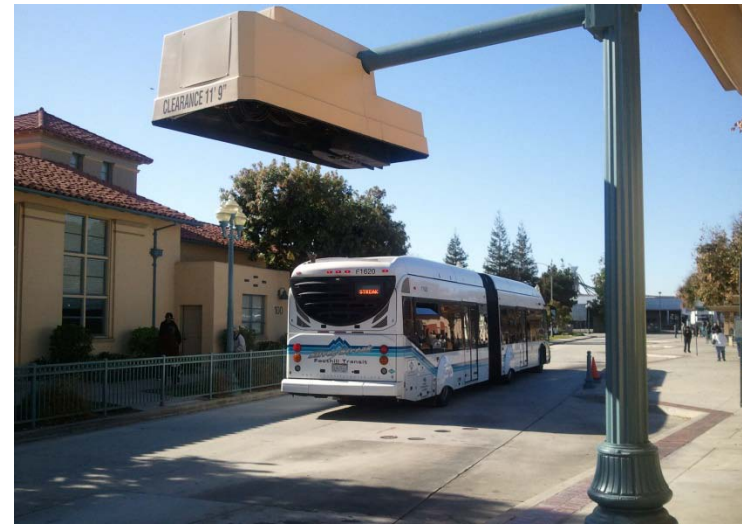
Figure 17-3: Electric bus charging station at the Pomona Transit Center for Foothill Transit
